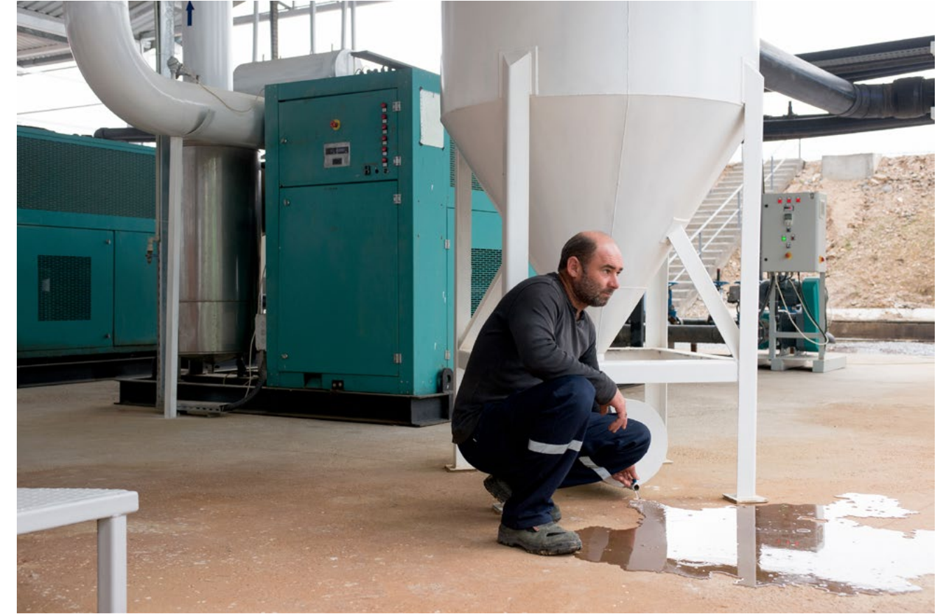
Biogas is produced by the natural fermentation of 450 tonnes of animal manure each day and covers the needs of 5,500 people with 2,4 MW daily electricity production. © Mathias Depardon pour l'Agence Française de Développement
